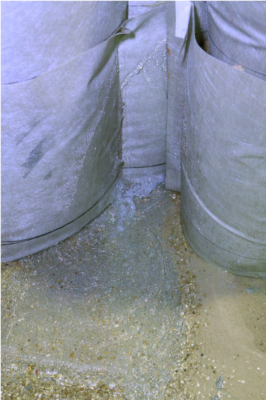
Figure 58. Close up of flow through joint in Geocell unit.
