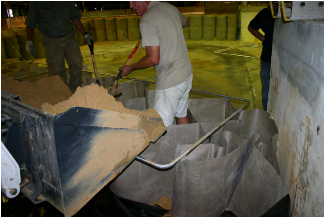
Figure 15. The extra cells where the final length angles into the wingwall will be removed with a box cutter.
