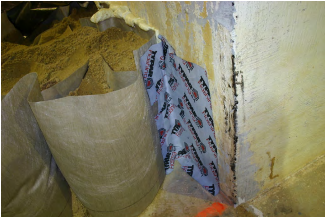
Figure 12. Flashing and expanding foam sealant were used to seal the Geocells to the wingwall.
