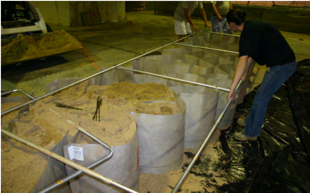
Figure 13. To fit the Geocells around a 63 deg. angle, the first cells are filled for a straight connection then the frame and remaining cells are turned to the desired angle.
