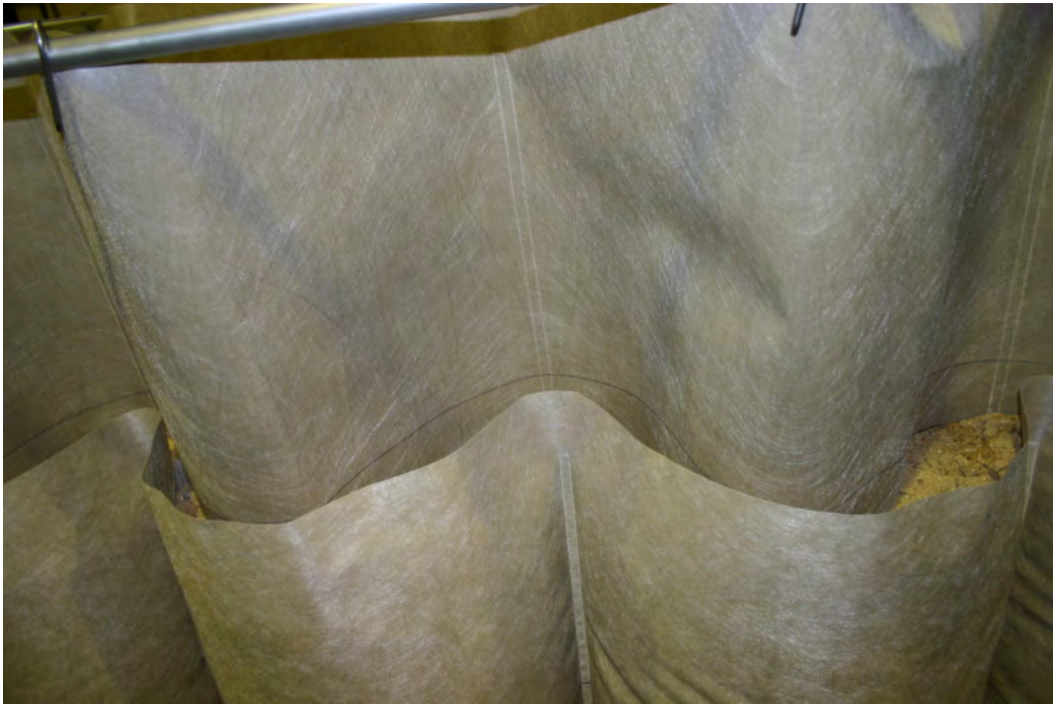
Figure 17. A line near the base of each Geocell matches up with the overlap of the outer wall of the first layer.
