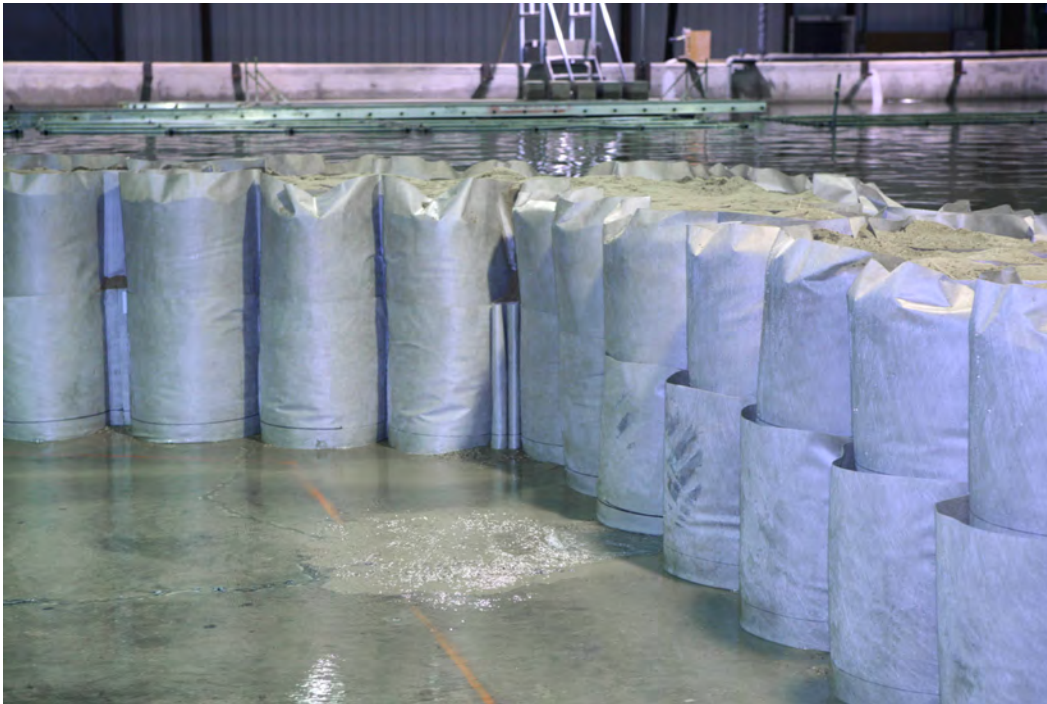
Figure 57. Seepage flow through joint in barrier near the angled Geocell unit.
