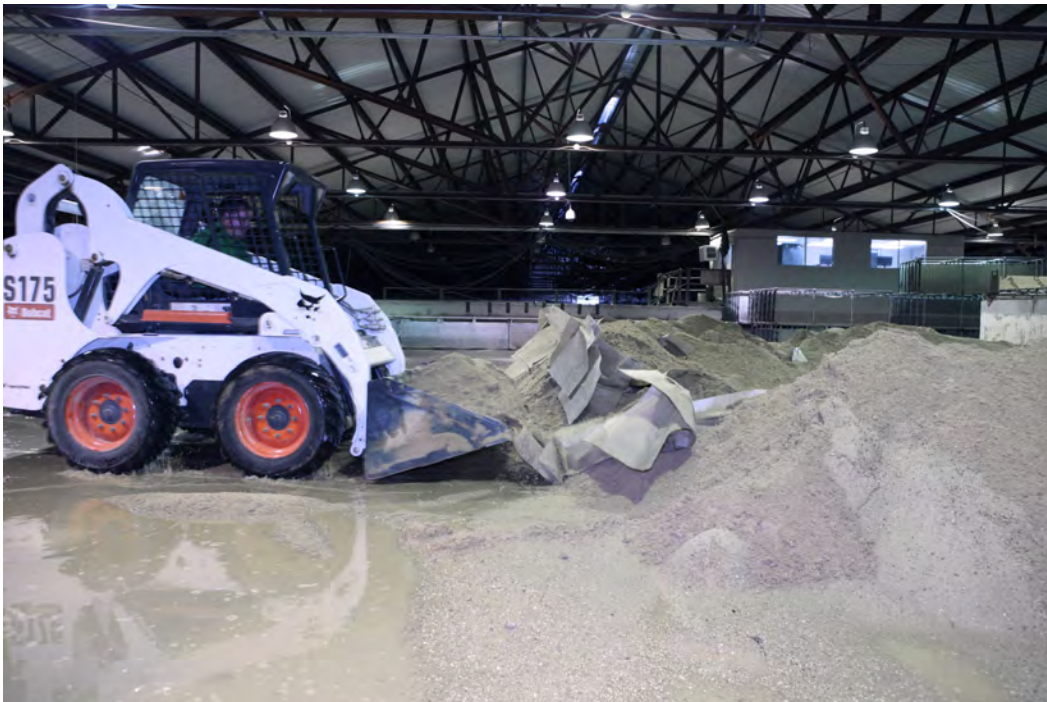
Figure 62. Sand is removed with front-end loader from each side of the barrier.
