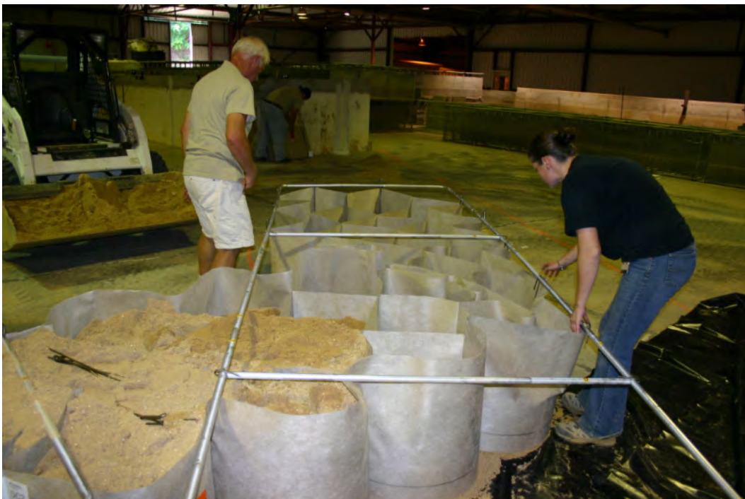
Figure 14. The frame and remaining cells have been turned to fit the designated layout.
