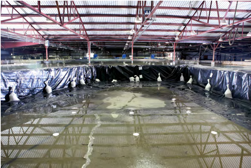
Figure 21. Sandbags were used to anchor the plastic sheeting on the inside of the barrier.
